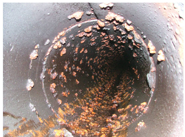
Figure 2: Corrosion at defects in the internal coating
